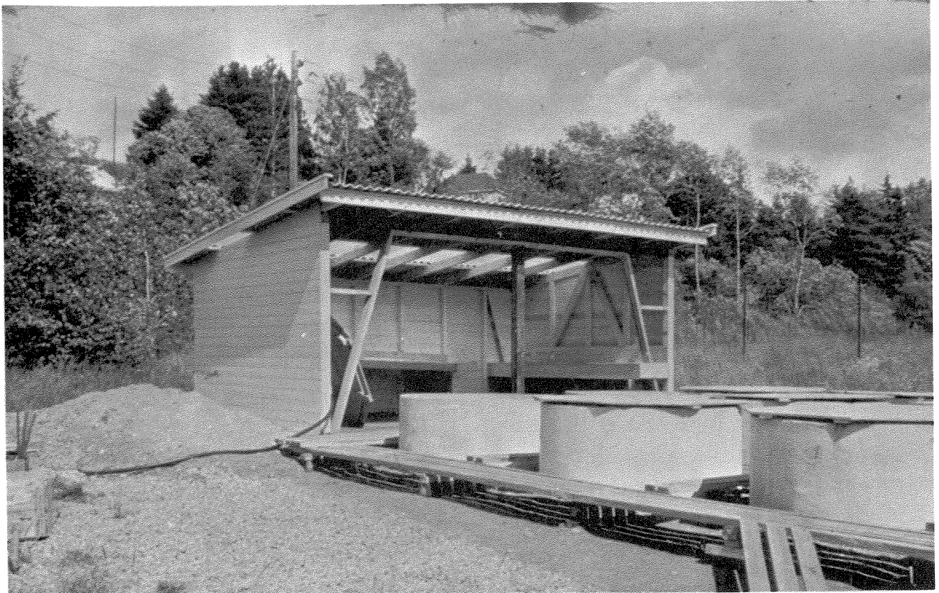
FIGURE 4 THE CONCRETE TANKS OF THE WELL SYSTEM.
