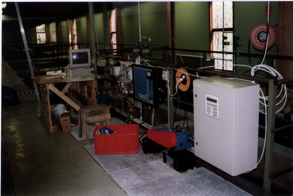
Figure 4. Coagulant Dosing Control unit at Bårilidalen WWTP
