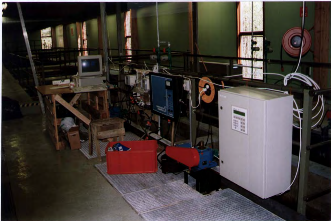
Figure 4. Coagulant Dosing Control unit at Bårlidalen WWTP
