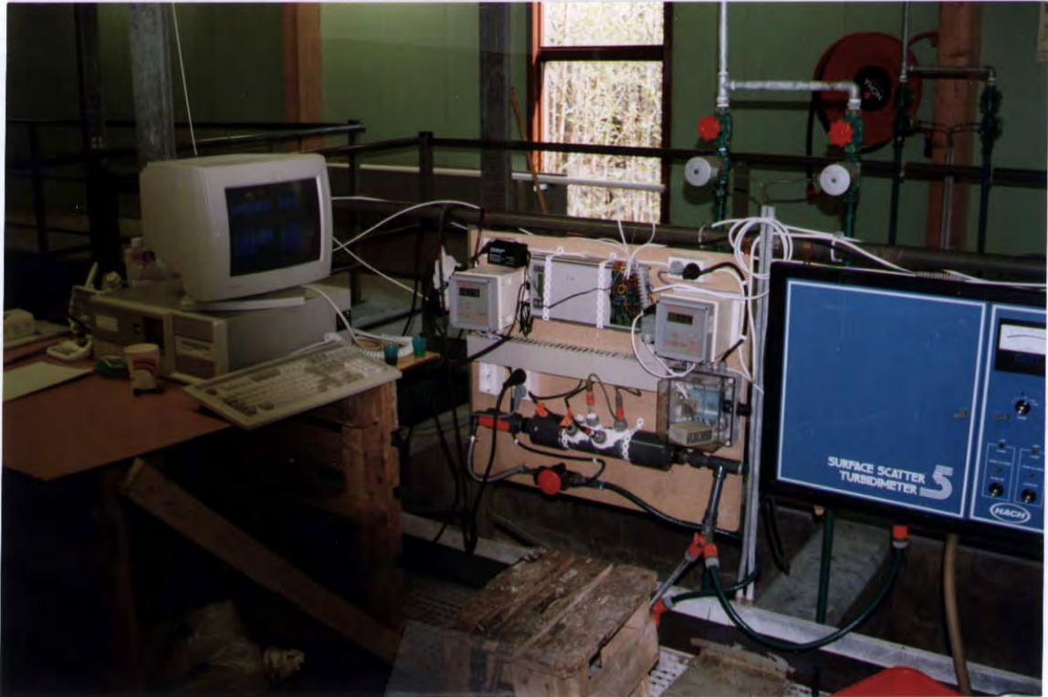
Figure 3. On-line water quality monitoring system at Bårlidalen WWTP
