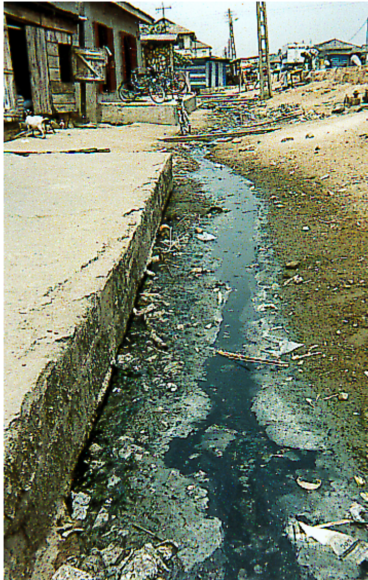
Figure 6. Open sewer in the drainage system in Nsawam, the Capital of South Akwapim District Eastern region -. This city was also suggested by MLGRD as a relevant pilot site area
