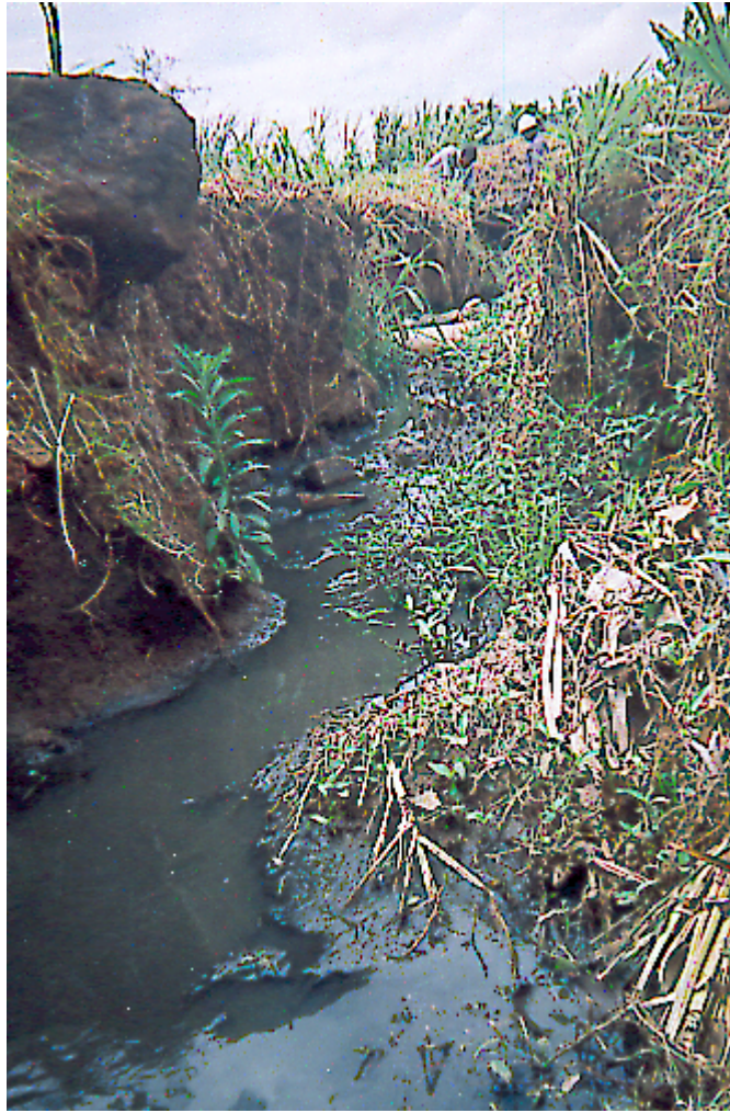
B.5 Sewage stream from broken pipeline
