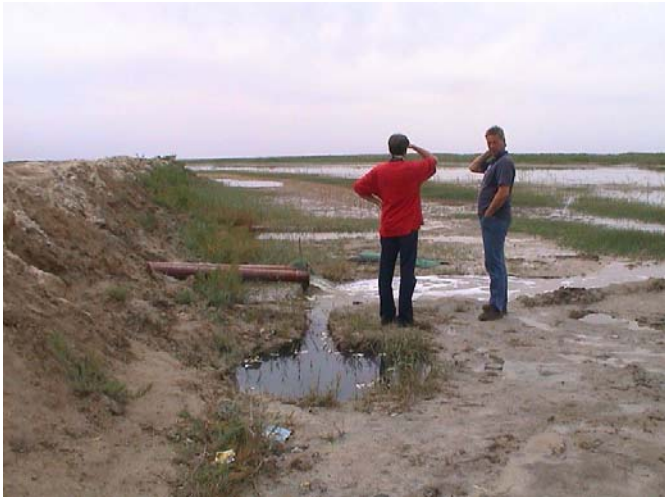
Figure 3.9 Discharge from sedimentation basin
