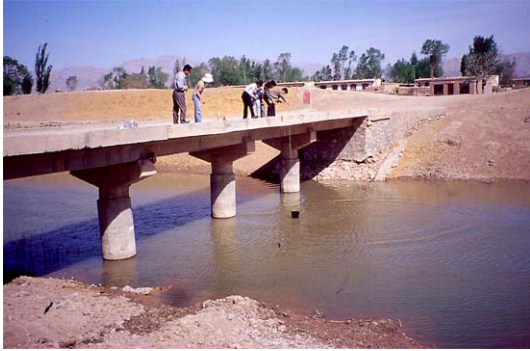
Main drainage canal, monitoring station no. 2, Sizhi Bridge
