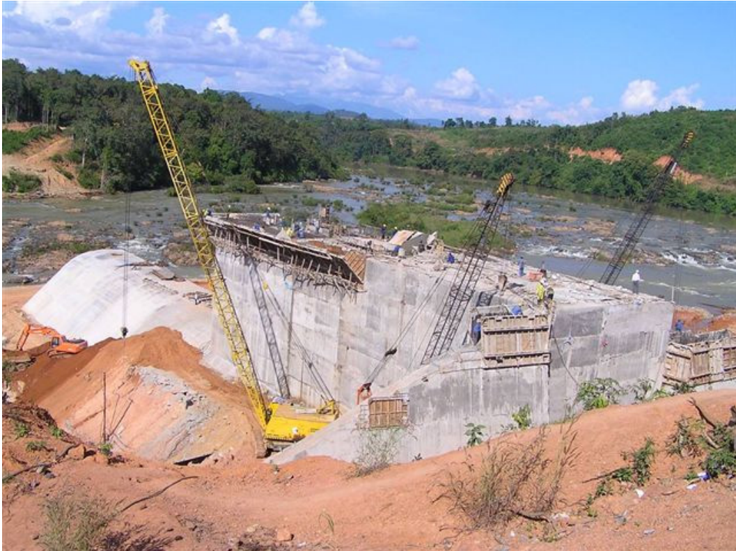
Figure 13-8 From the construction of the Se San 4A Re-regulation reservoir. Photo EVN 2006.
