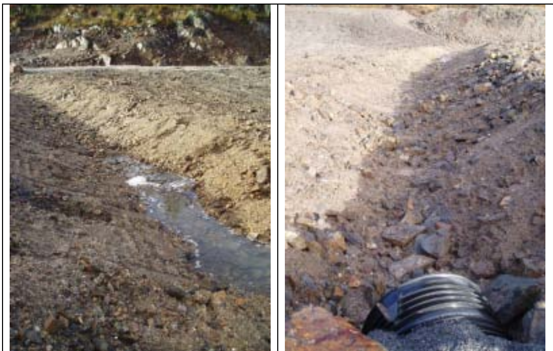
Figure 15. Open ditch across M17 on November 17, 2009. The stream in the picture to the left was supposed to cross the fill and enter the pipe in the picture to the right. Instead, it runs into the fill halfway over.
