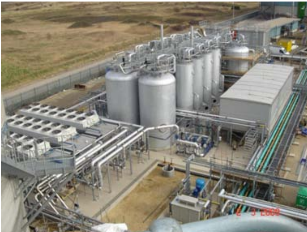
Figure 34. A photo of Bran Sands sludge treatment plant in UK (Aker Solutions 2009) using Cambi ® THP process (in the middle of photo) for pre-treatment to enhance biogas production (in commissioning 2009)
