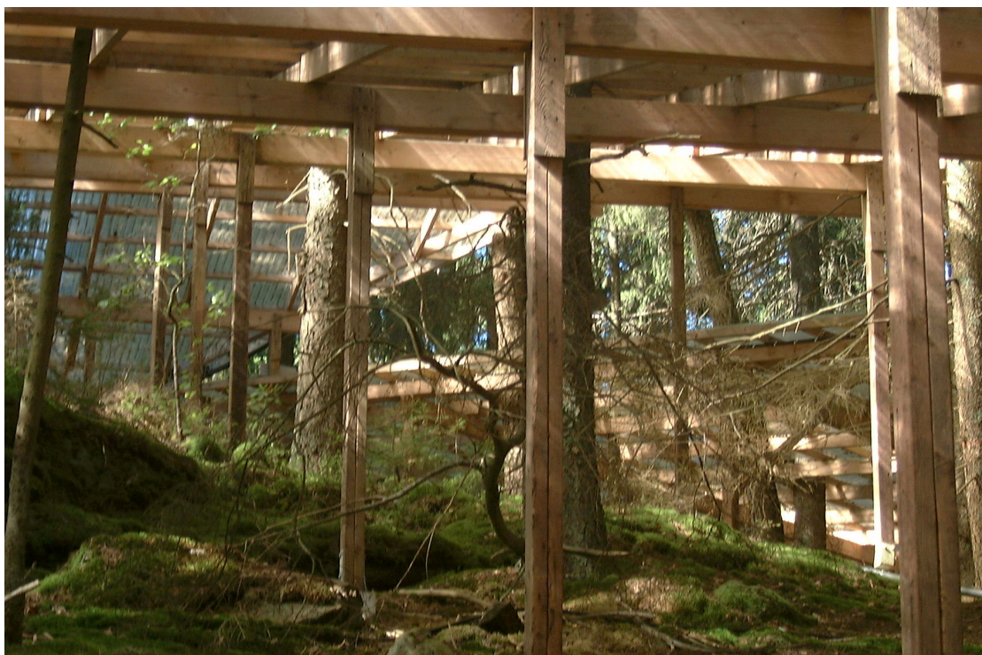
A plastic roof was constructed over the catchment G1 at Gårdsjön, Sweden in 1991.
