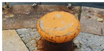
Figure 16. A weathered mooring. Photo: Amy Lusher
