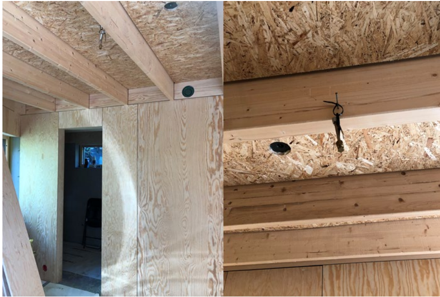
Figure 15. The sampling site with highest concentrations of \alpha - and \beta -pinene. The untreated natural wood materials act as a source for pinene emission to this indoor environment.
