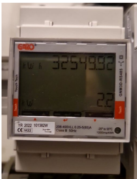
Figure 6. Photo of the electricity meter measuring energy use in kWh for the SUPI aquaponic system at Natur VGS.
