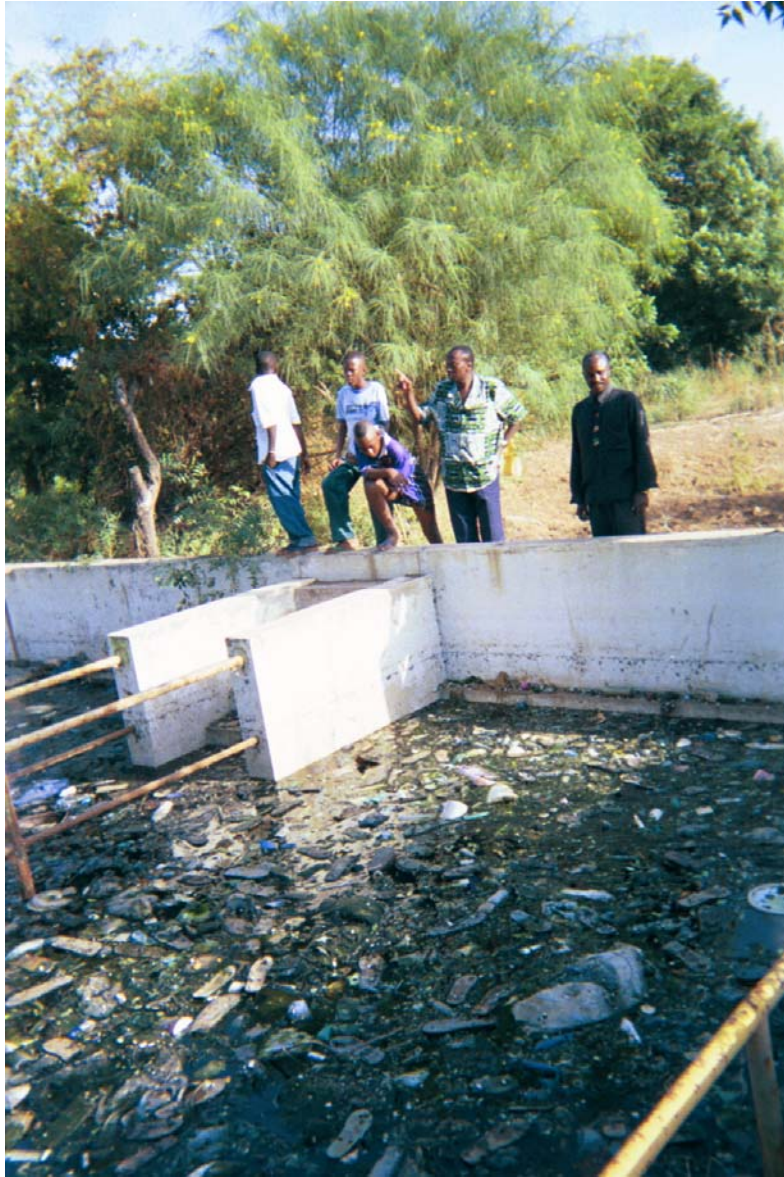
Figure 6. Holding basin for sewage from l'école polytechnique in Thiès
