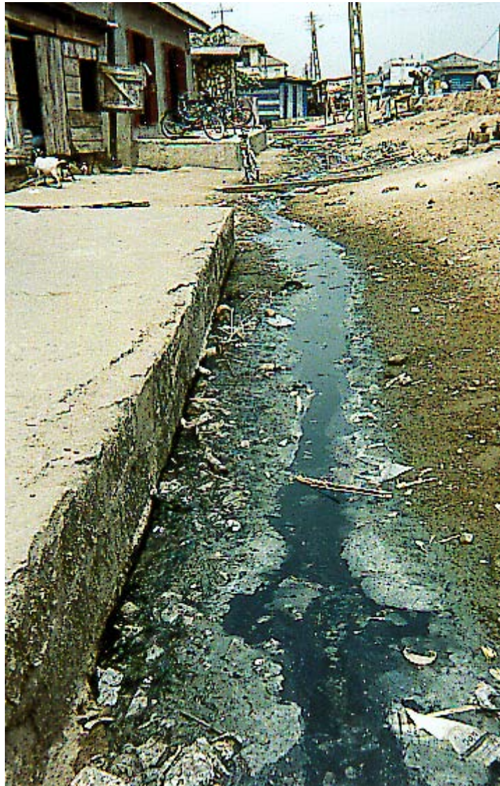
Figure 6. Open sewer in the drainage system in Nsawam, the Capital of South Akwapim District Eastern region -. This city was also suggested by MLGRD as a relevant pilot site area
