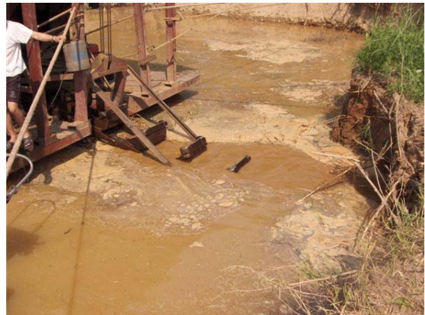
4. Digging down to 1.5 m below the water surface, and 1 m above the water surface
