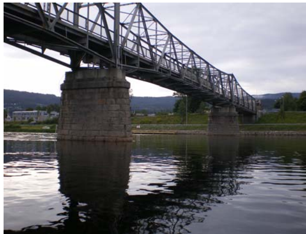
Figure 2-1. RID programme site on the Drammenselva River.
