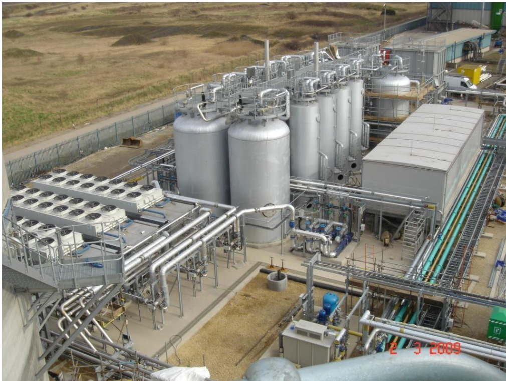
Figure 34. A photo of Bran Sands sludge treatment plant in UK (Aker Solutions 2009) using Cambi ® THP process (in the middle of photo) for pre-treatment to enhance biogas production (in commissioning 2009)
