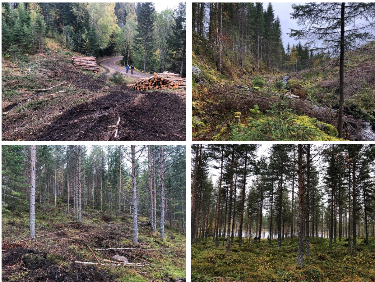
Figure 2: Recent forestry activity in the Glitre catchment. Top left: clear cut near the northernmost point of Glitrevann (October 2019). Top right: close to Guritjernsbekken (within the last 5 years). Bottom left: a recently thinned parcel close to Gjøssjøbekken (2019). Bottom right: a half-mature parcel. Source: NIVA
