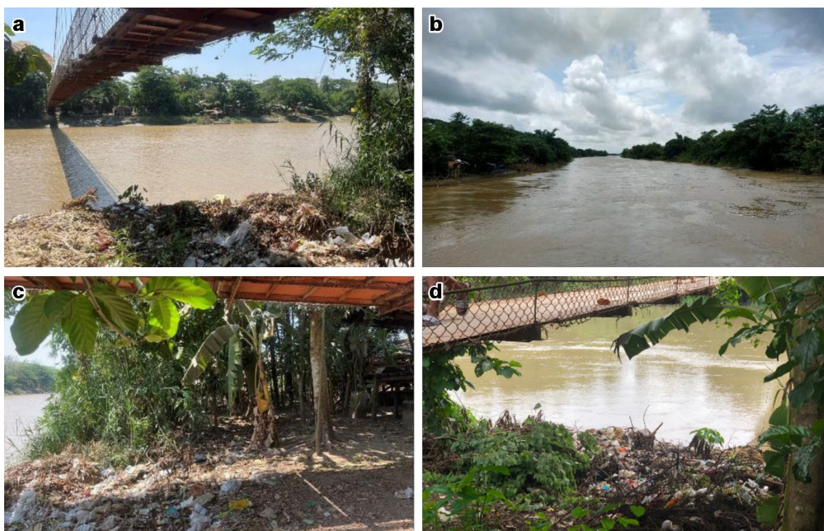
Figure 3.4. Location 3 and the Kyauk Tan Bridge. The bridge and river are depicted in a and b. Waste dumped and accumulating along the riverbank and under the bridge is visible in a, c, and d. (Source: photos a, b, c Kyaw Min San 2023, photo d, May Phoo 2023).
